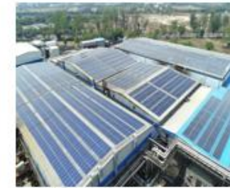
Rooftop Solar in Hapur
