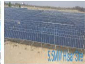
Ground mounted Solar by MIL Rohad, in Budak
